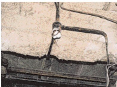
Sprayed asbestos on steelwork (typically amosite)
