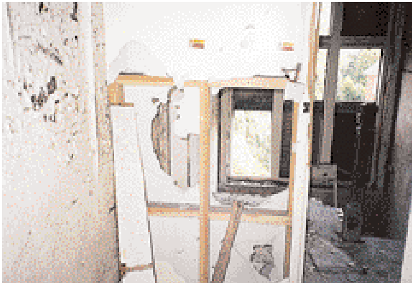
Damaged asbestos insulating board (AIB) panels containing amosite (brown asbestos)
