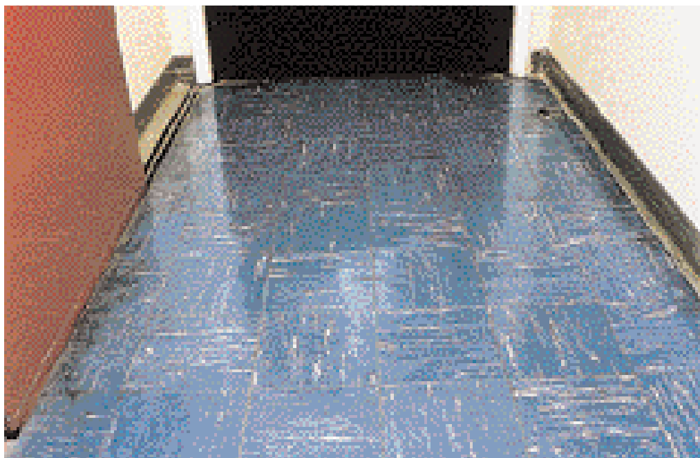
Asbestos-containing vinyl floor tiles (chrysotile – white asbestos)
